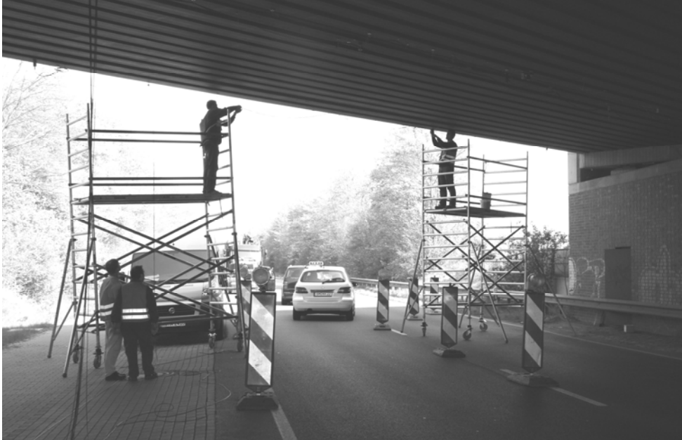
Figure 5: View underneath the Erfittal Bridge on measurement day 2. Closed lane to the right, paved “green strip” and bicycle/pedestrian lane to the left
